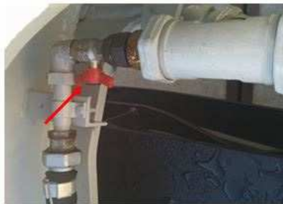
Absperrhahn in offener Position
